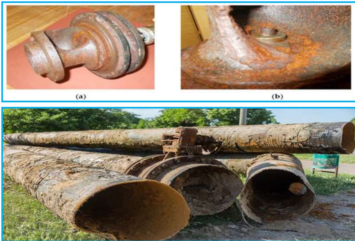
Fig: Damage of GI Pipe by physical and chemical means
