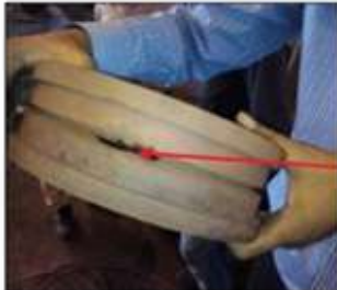
4 : Push-through seal valve seat damaged by sharp debris pushed through while closing
