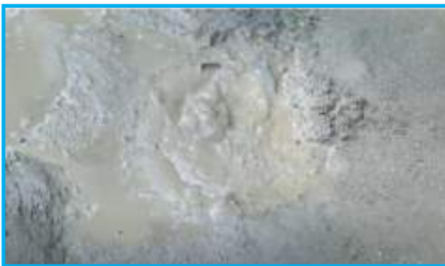
Leakage in Distribution Pipeline
