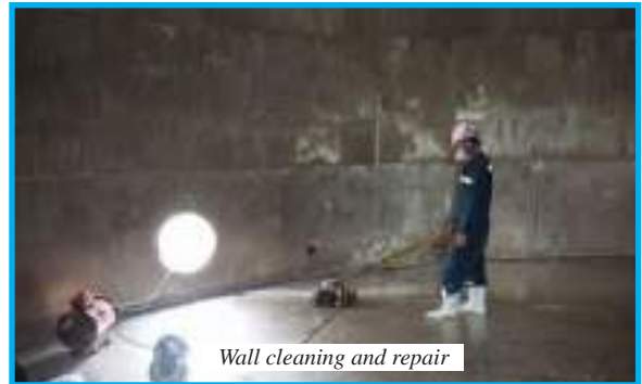
Drain the water from reservoir
