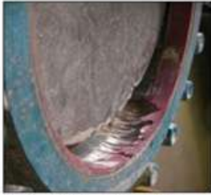
1 : Incomplete closure caused major damage of perimeter seal and body
