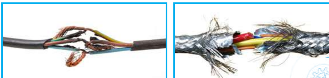
Fig: Damage of 3 phase wiring of a Centrifugal Motor
