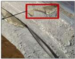
7 : Hard scaling in body of a perimeter seal valve used in nickel slurry
