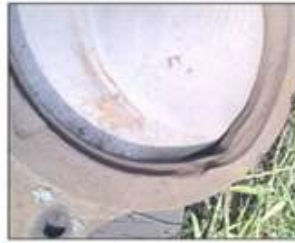
8 : Erosive wear on valve body caused by abrasive slurry
