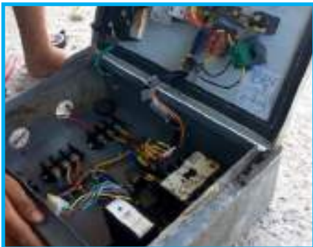
Inspection of starter box
