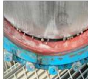
6 : Particles stuck between gate and perimeter seal in valve preventing closure
