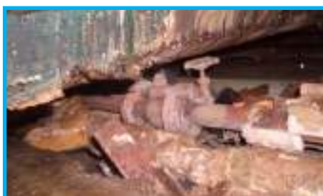
Corroded pipe section, highlighting the corrosion damage
