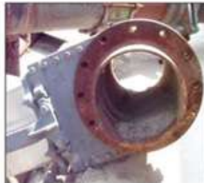
5 : Slurry deposition by dewatering and hardening in valve body and pipeline
