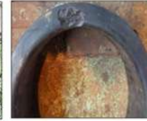
9 : Push-through seal valve seat damaged in face area by elastomer deterioration.
